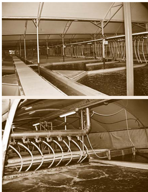
Fig. 63.17 Water channels and air distribution system. Air-flow rate is controlled by regulating air-blower frequency using readings of oxygen concentration in the fish tank
